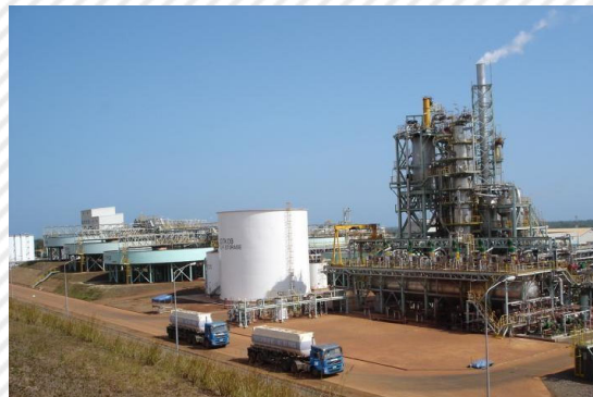
Coral Bay Nickel plant in the Philippines (Photograph courtesy of Sumitomo Metal Mining Co., Ltd.)
