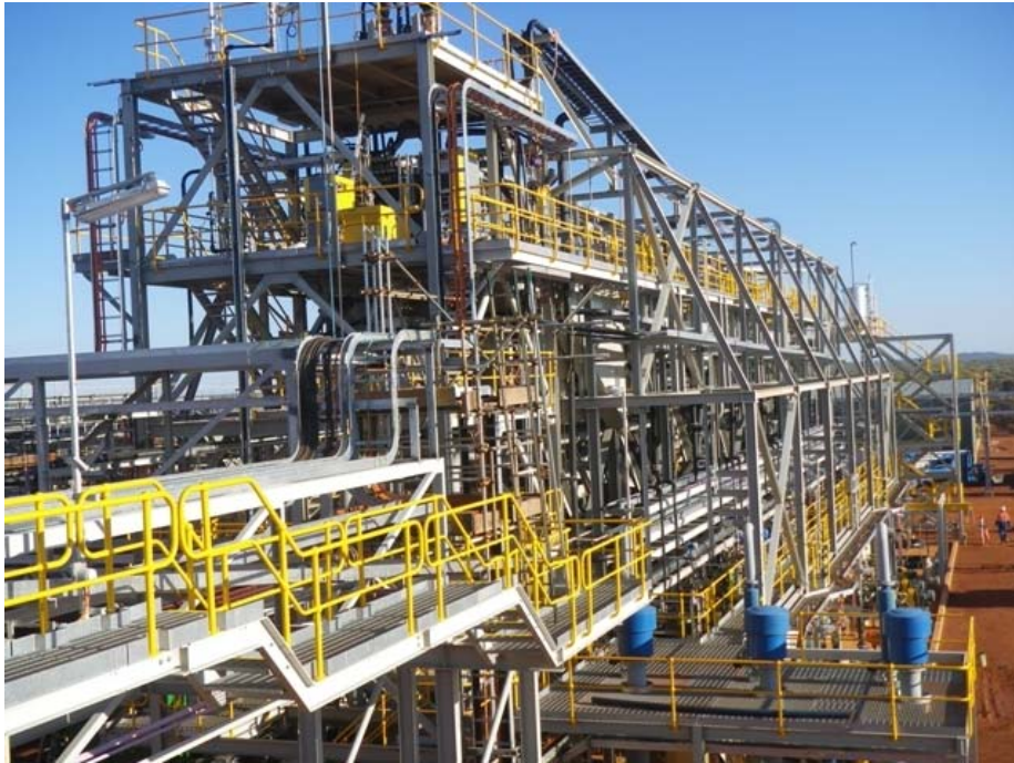
Mount Weld Rare Earths Concentration Plant
