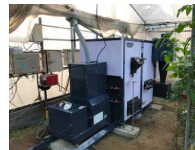
Biomass boiler installed at banana plantation
