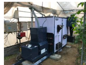
Biomass boiler installed at banana plantation
